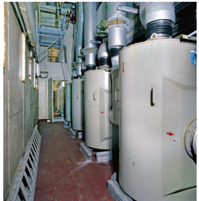
Filter room created in the void between the inner and outer shell of the bunker during the 1980s refit.
